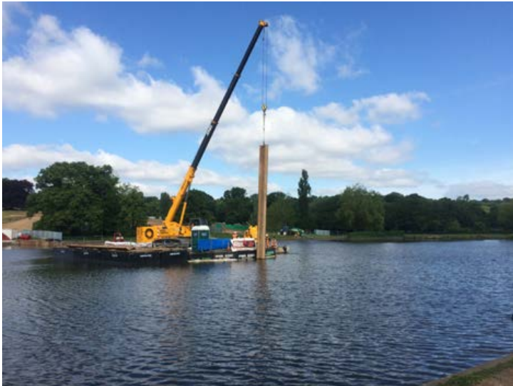
Picture 3 - The crane is floated on pontoons alongside the rig, to feed the sheet metal piles.
