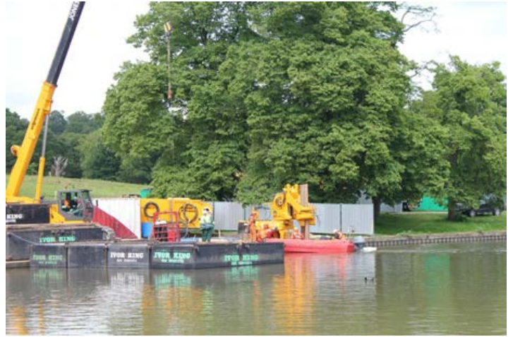
Picture 2 - The piling rig pushing the sheet-metal piles into place using a silent vibration-less technique.
